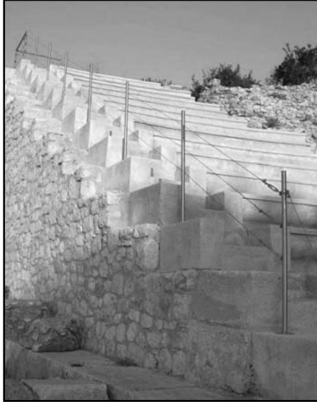
Fig. 14: Theatre, steel posts and fencing along the seats
