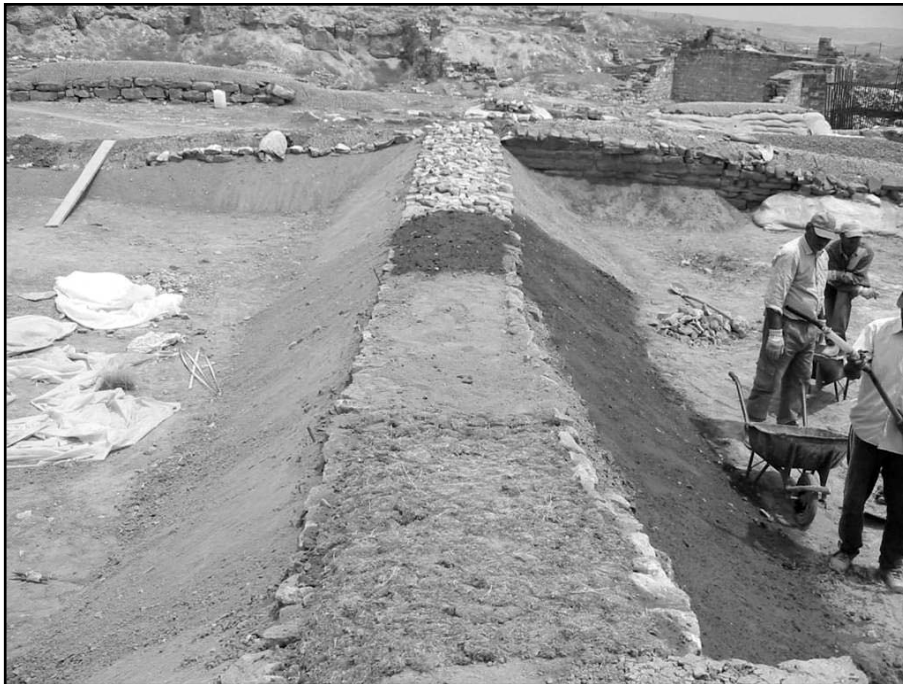
Fig. 15: Sand-earthen slopes at angle of repose in Terrace Building and variety of wall cappings
